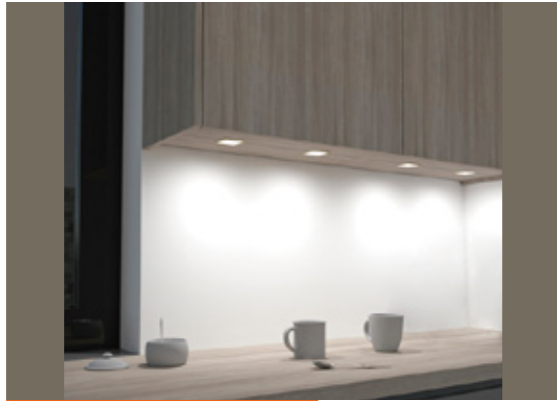
Under Cabinet Lighting
